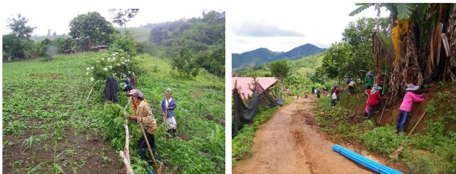
Community volunteers supporting construction of the piping system in Ban Huay Moo
