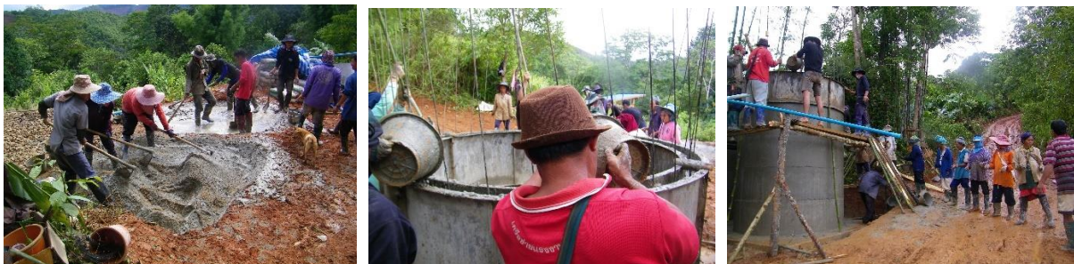
Construction of the two storage tanks by KHT team and community volunteers in Ban Yod Pai
