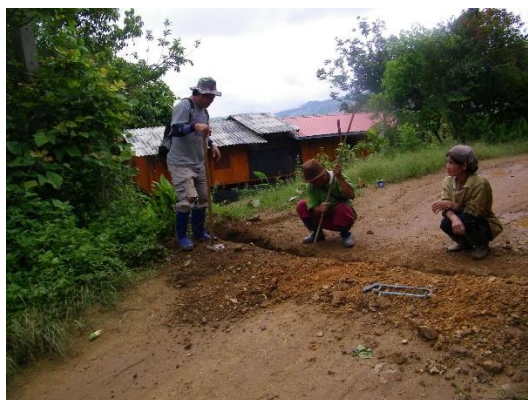
KHT Construction Manager, Aka (left), working with community volunteers on the pipeline in Ban Yod Pai
