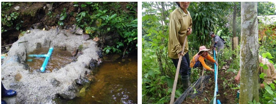
Water source collection point (left); KHT team joining the new and existing pipelines (right)
